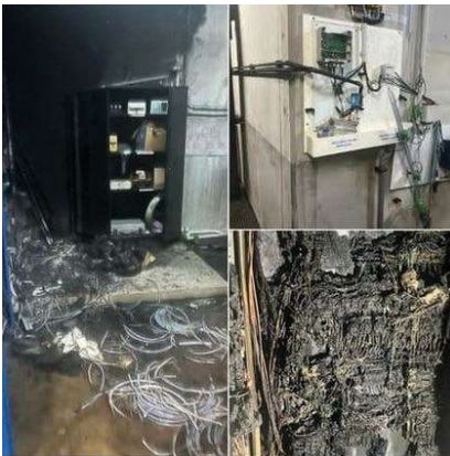
Draveil (Essonne) 1 st /2 nd July: the electrical system at the leisure centre set alight
